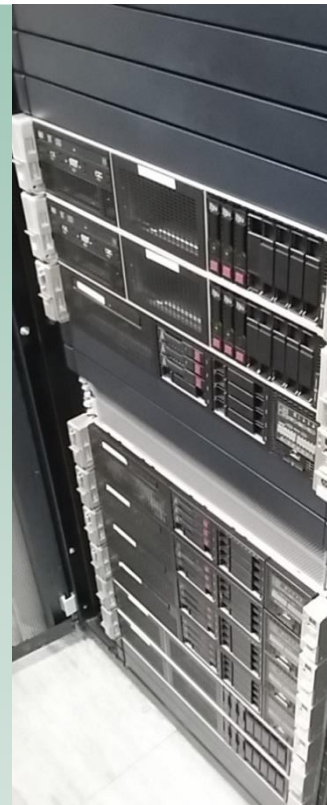
Above: photograph of the SVO Hardware installed in WPD's Central Server Room.
