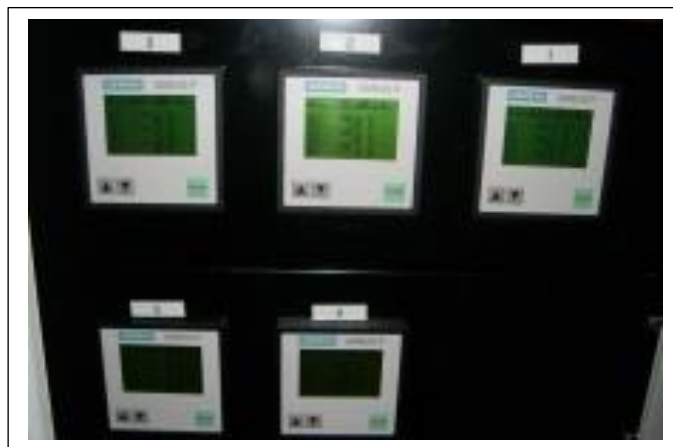
Fig. 3 Sub-station monitoring Meters
