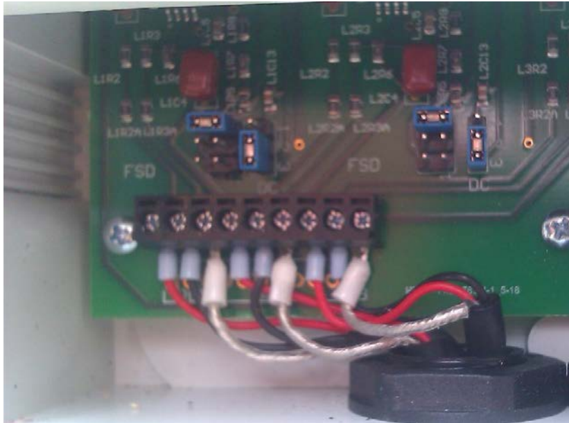
Image 6: Small wiring connections
