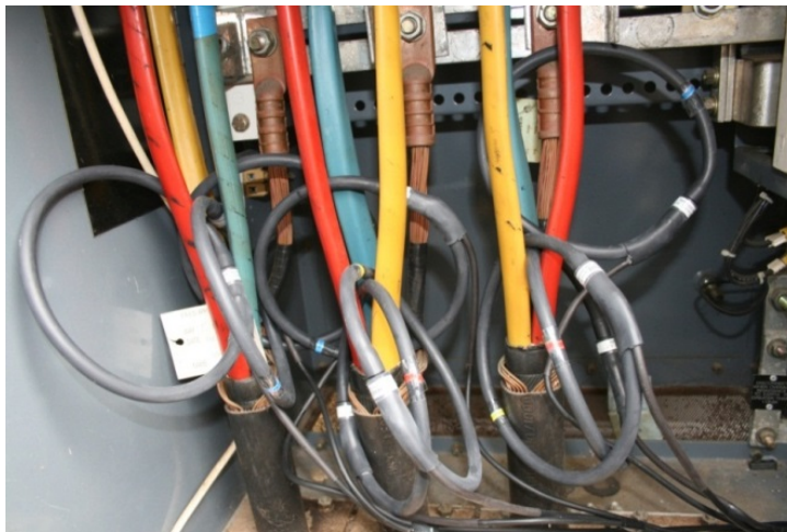
Picture 2: Rogowski coils around LV cable cores
