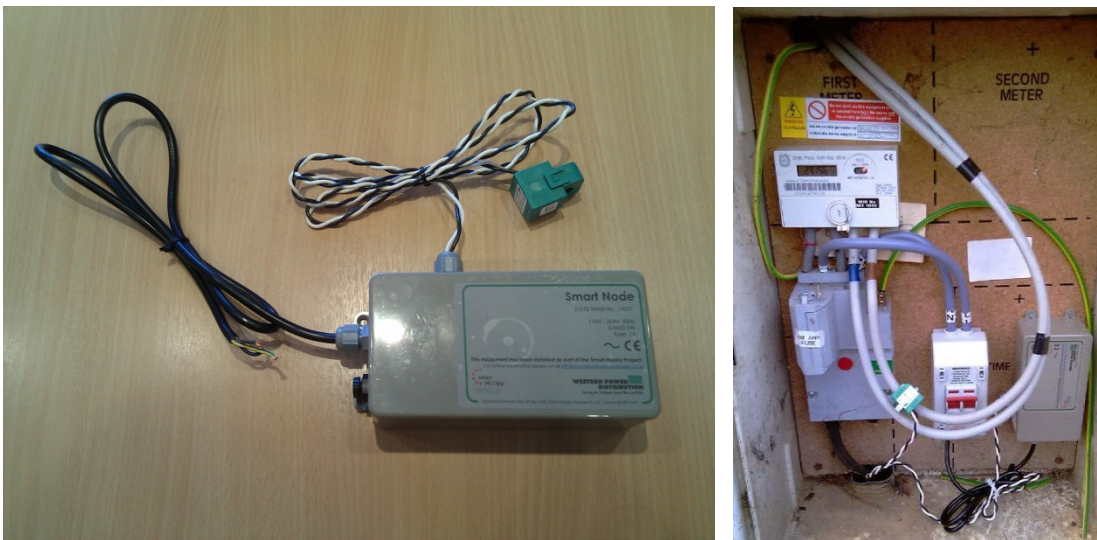
Images 7 & 8: Smart Node with power lead and CT (left) and installed in outside meter box with dual pole isolator switch (Right).
