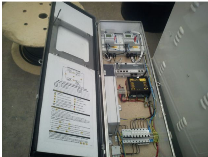
Image 5: Example of power meters mounted on top of Rogowski Interface units
