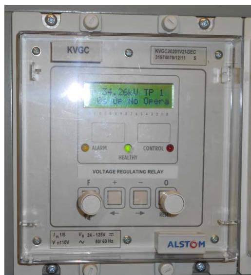
Figure 4-6: Picture of KVGC202 Relay
