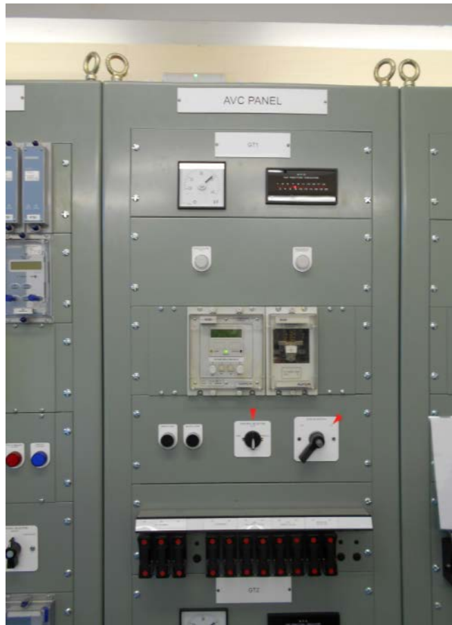
Figure 4-7: Picture of KVC202 inside Panel
