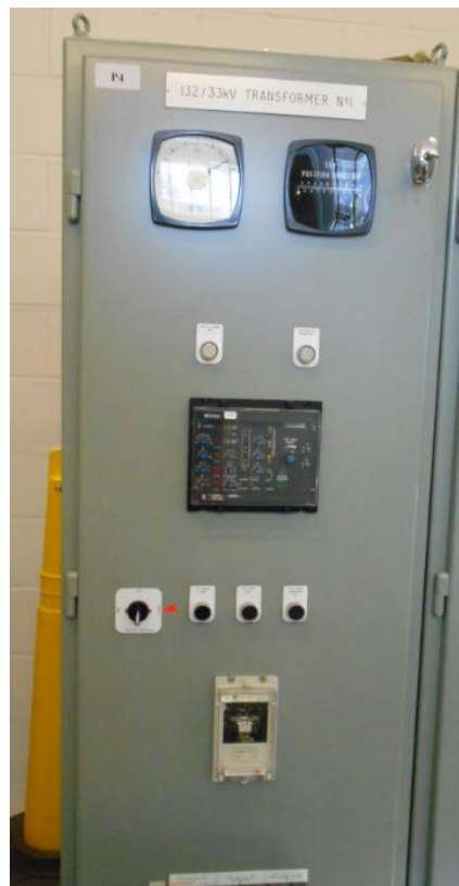
Figure 4-2: Picture of MVGC01 inside Panel
