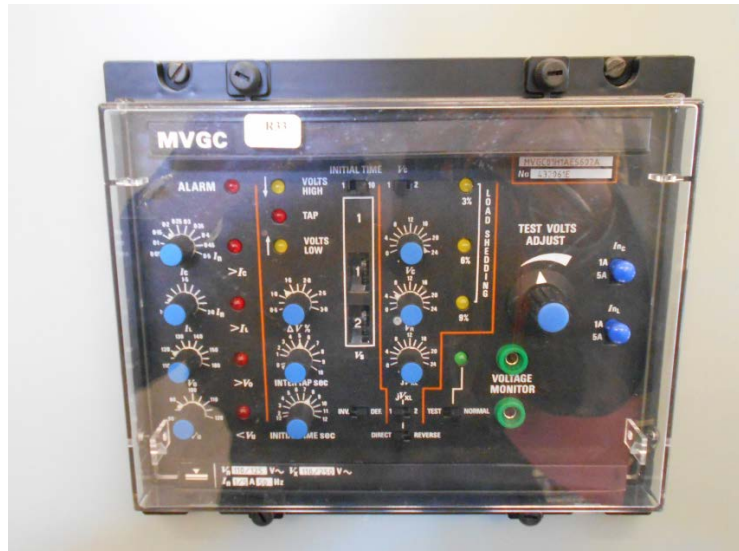
Figure 4-1: Picture of an installed MVGC01
